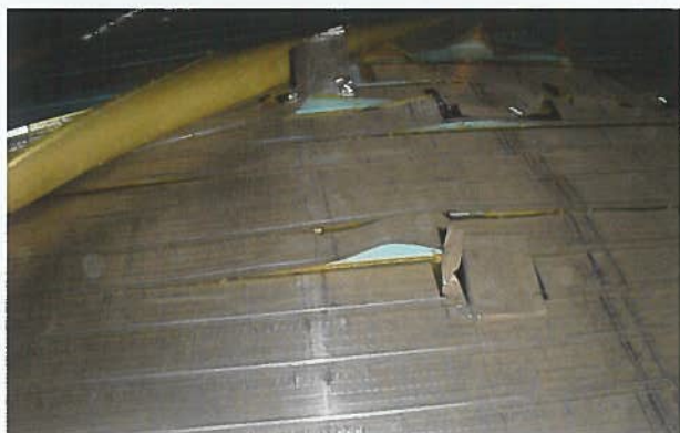
Figure 1. Typical problems seen in the insulation systems.
