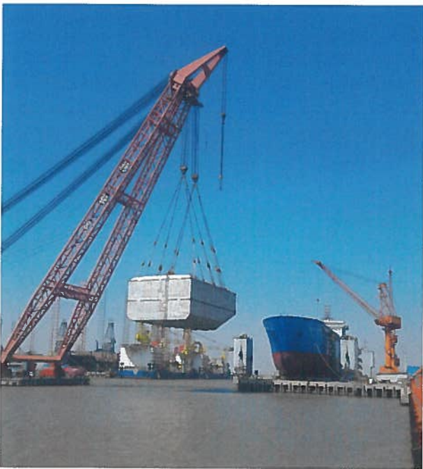
Figure 4. LNT Fuel-Box – the tank is constructed in parallel with secondary barrier installation.
